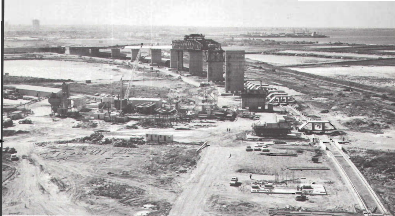
The West Gate Bridge in March 1970 showing piers under construction, a pre-casting factory, pre-cast units alongside bridge, and an erection truss.
